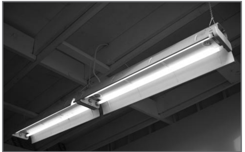
Old T12 fixtures at BRING's Planet Improvement Center were converted to use more energy efficient T8 ballasts and tubes. By not buying new fixtures, we saved the energy and resources it would have taken to make new ones, and we reduced the energy we need for lighting.
