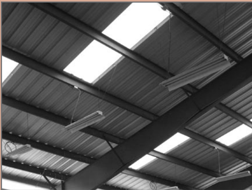
Plastic panels can bring light into a large space. At BRING's retail outlet, the covered shopping area not only protects materials from the weather, it also lets light fill every corner. The design is so efficient, it is only during the winter months that we need to augment the natural light with artificial light.
